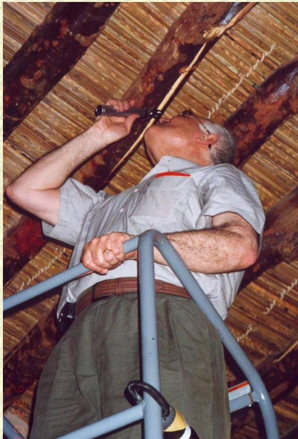
Diagnosis of cracks
