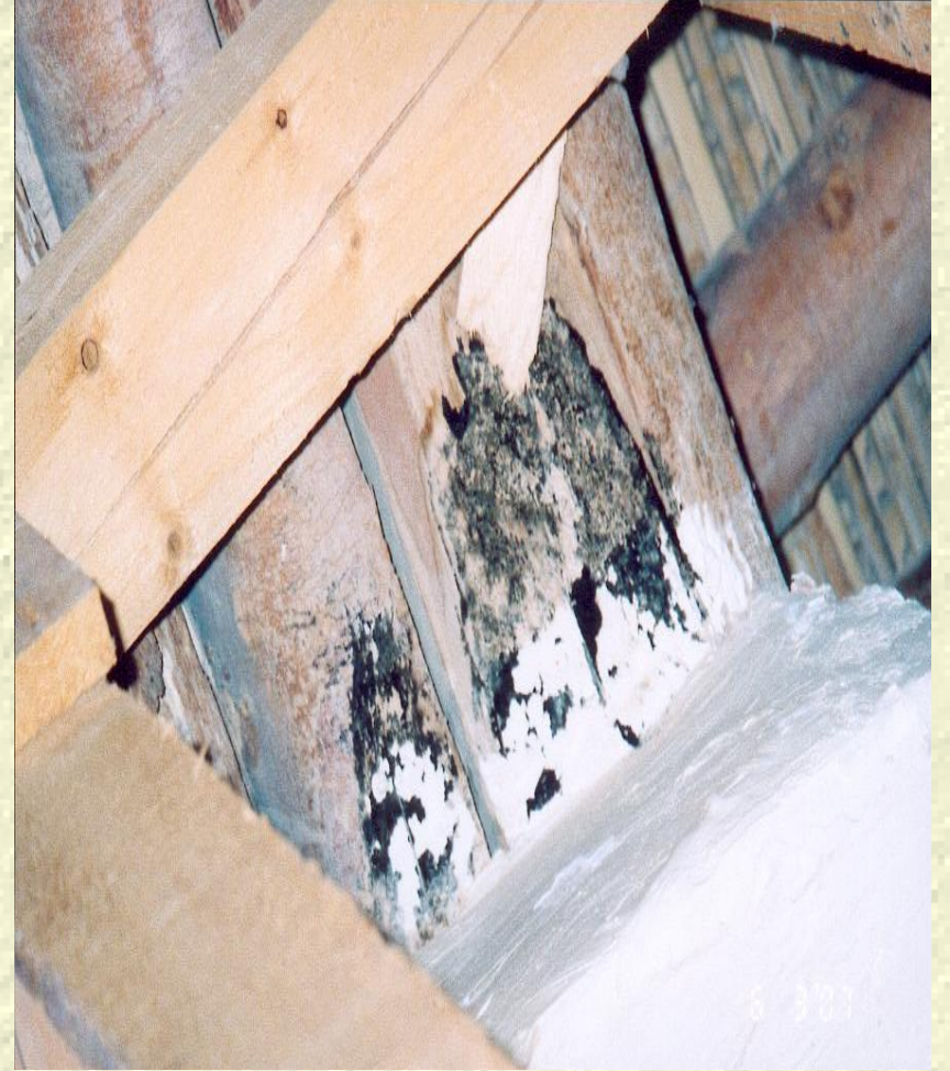
Decayed wood in roof by fungi & termites
