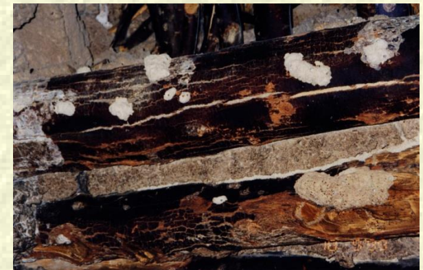
Deterioration in wooden roof- insects nest
