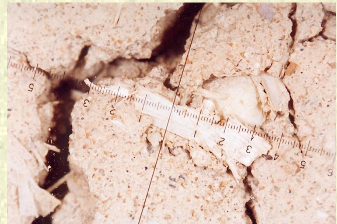
Cracks by Dermaphot – magnified 1/20
